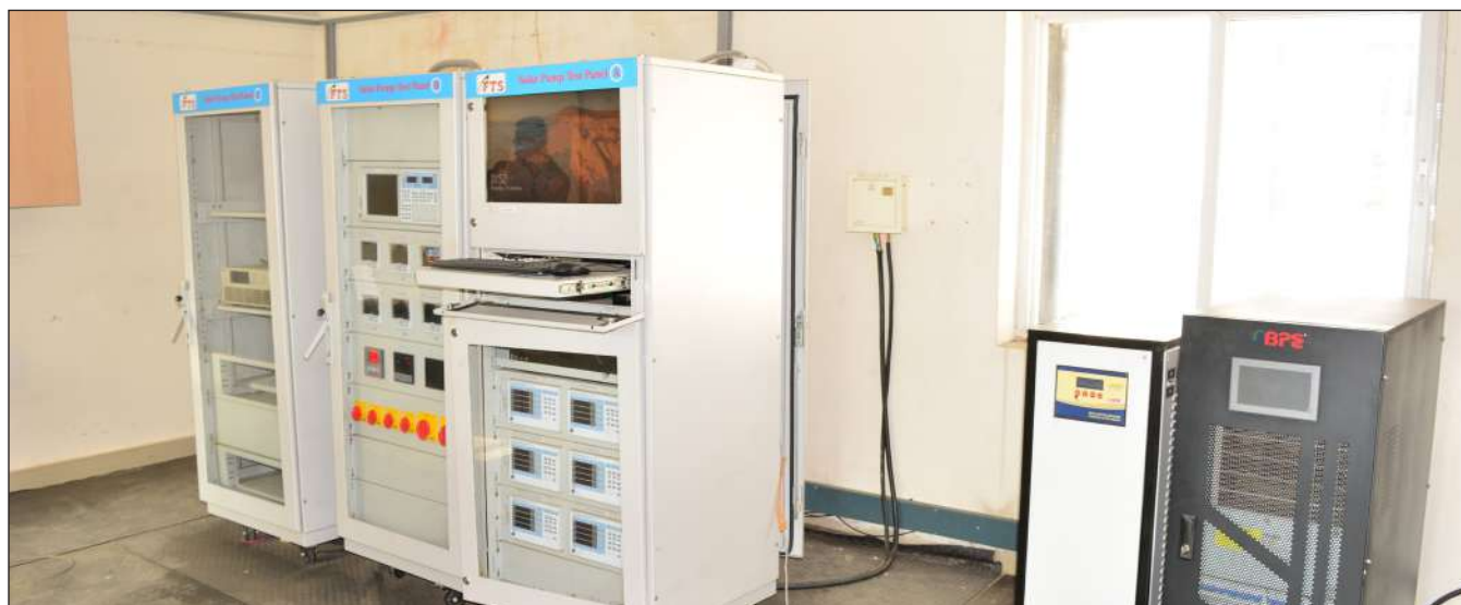
Figure 2.10: Solar Water Pump Test facility for up to 50 hp
